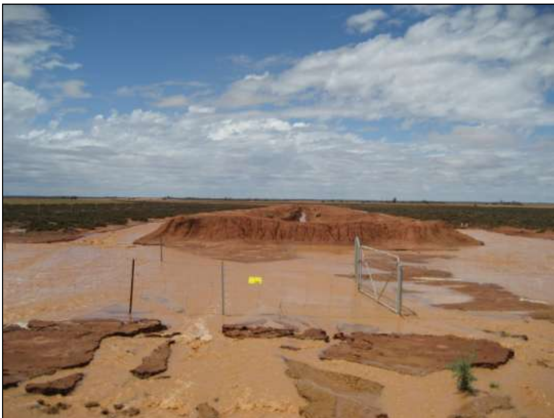
Fig 19: Putting the design to the test. Mongers 55 deep drain, standing up to a major flood event in February 2008. Notice that the surface water remains separated from the groundwater inside the drain.
